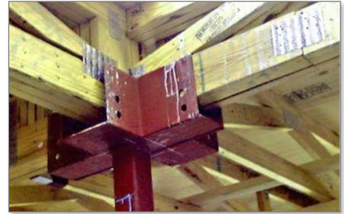
Building Code violation
