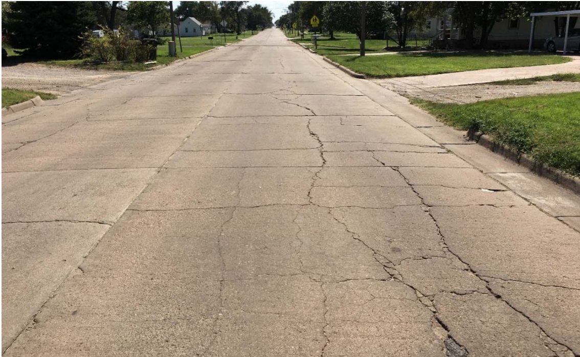
Figure 9: Image showing existing concrete deterioration on Lincoln St.
